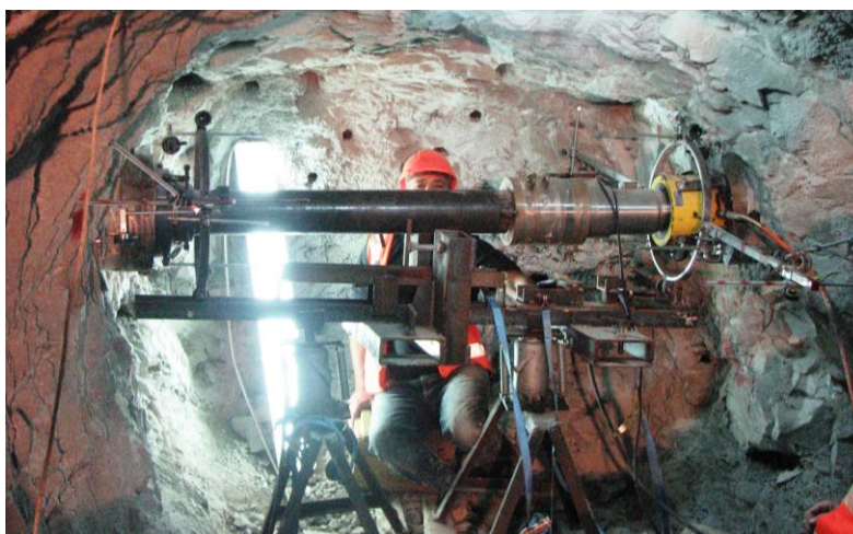
Fig. 6: Horizontal setting of the Plate Loading Test. (Performed by the Building and Infrastructure Testing Lab. Israel)
